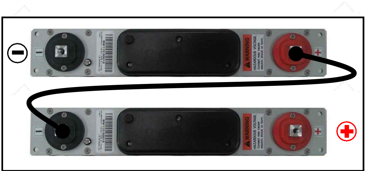
< Fig. 2 > Series Connection of Modules
